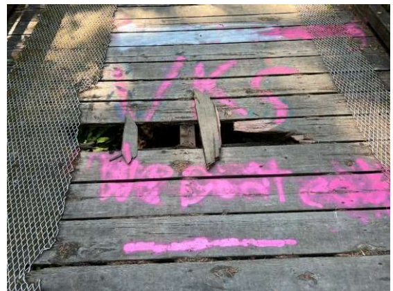
Photo 4: Deteriorated and broken decking.
