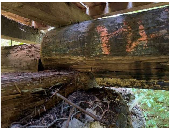
Photo 7: East log beam end at bent.
