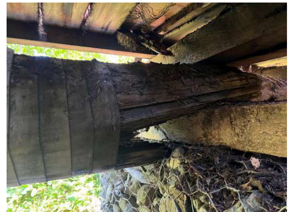
Photo 8: West log beam failure at bent.
