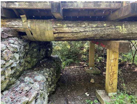
Photo 5: West log beam end at bent.
