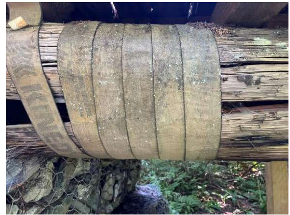
Photo 6: West log beam split at bent.
