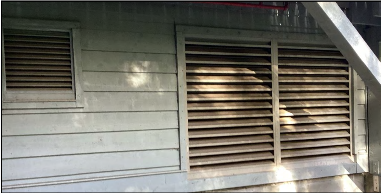
Image 6 - This image illustrates some of the HVAC venting that requires installation of 3 mm metal screen.
