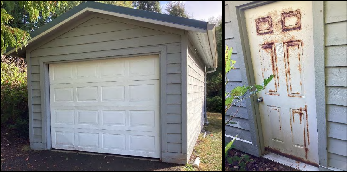
Image 13 & 14 – These images illustrate the condition of the doors on the storage garage.
