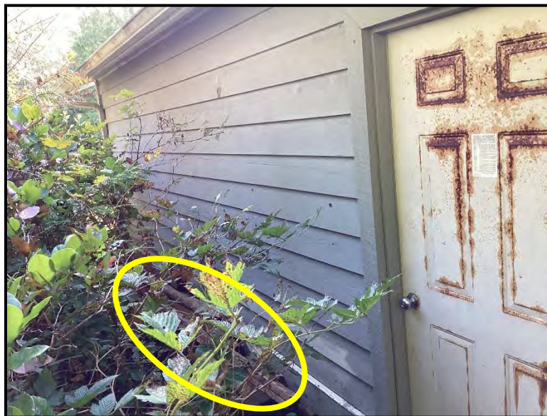
Image 15 – The yellow oval in this image illustrates the location of the combustible storage and vegetation growing within the Non-Combustible Zone of the storage garage.
